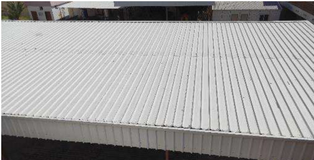
Eastern border of the proposed site for PV installations at Oqba bin Nafe' School
