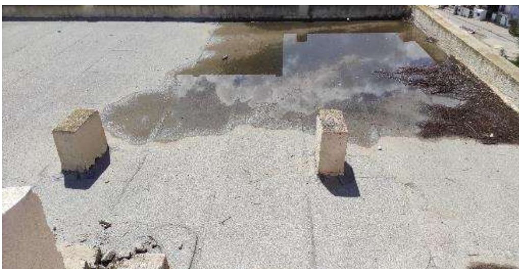
Southern border of the proposed site for PV installations at Oqba bin Nafe' School
