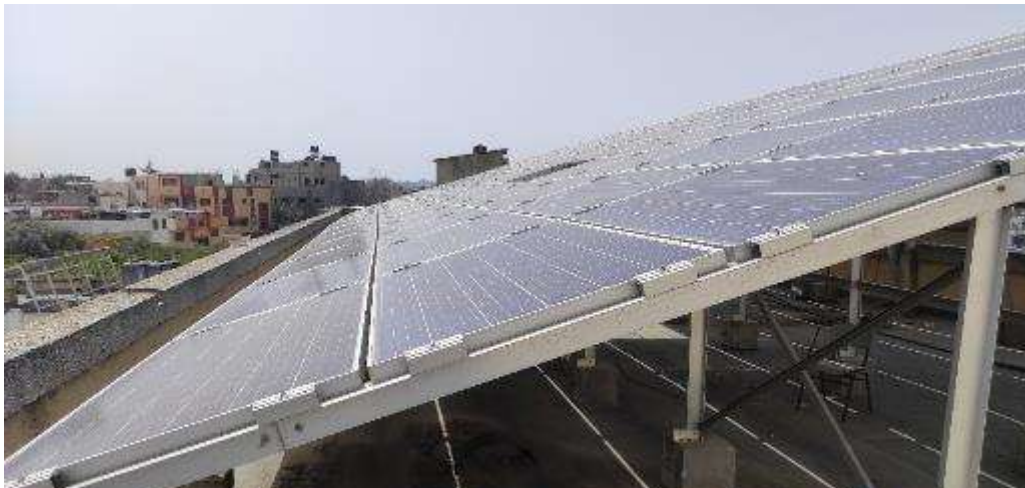
Proposed site for PV installations at Ashaymaa School (The MoEHE will remove this system to allow for the proposed system installation)
