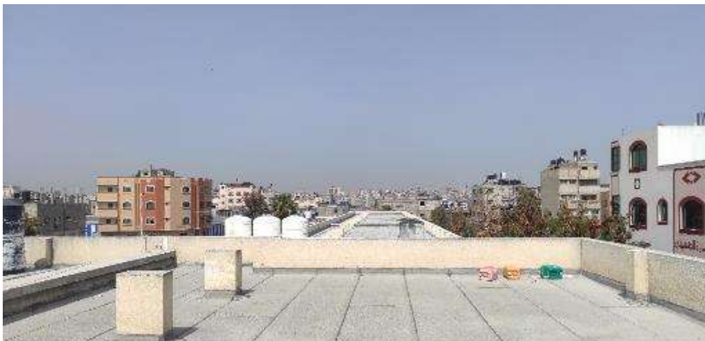
Western border of the proposed site for PV installations at Sumaya Bint Kheyat School (Ain Jalout School)
