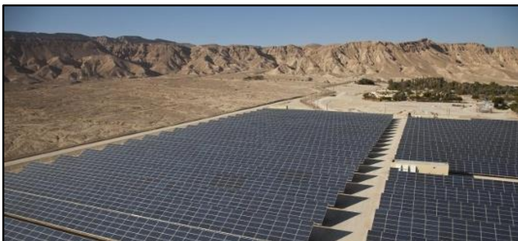
Figure 2: Typical PV Power Arrays Composed of PV Panels
